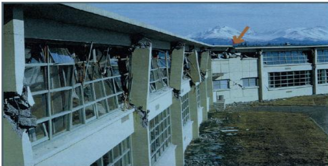
Fig 1. Damages Caused to the Roof Diaphragm at the Re-entrant Corner of West Anchorage High School, Alaska, during the 1964 earthquake
